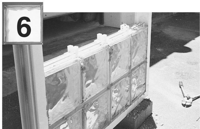
Repeat for second course using straight connectors with jamb connectors at each end.
