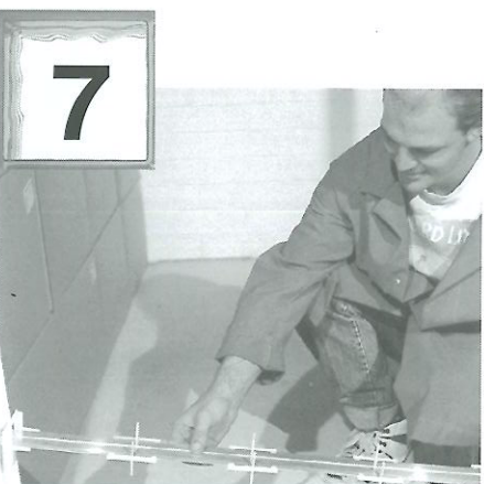
7 Place the stiffener bar, with connectors, onto the first row of glass blocks.
