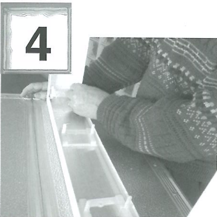
4 Place a cut "T" connector in the bottom corners of the frame on top of the sill infill, with the open end against the expansion material.
